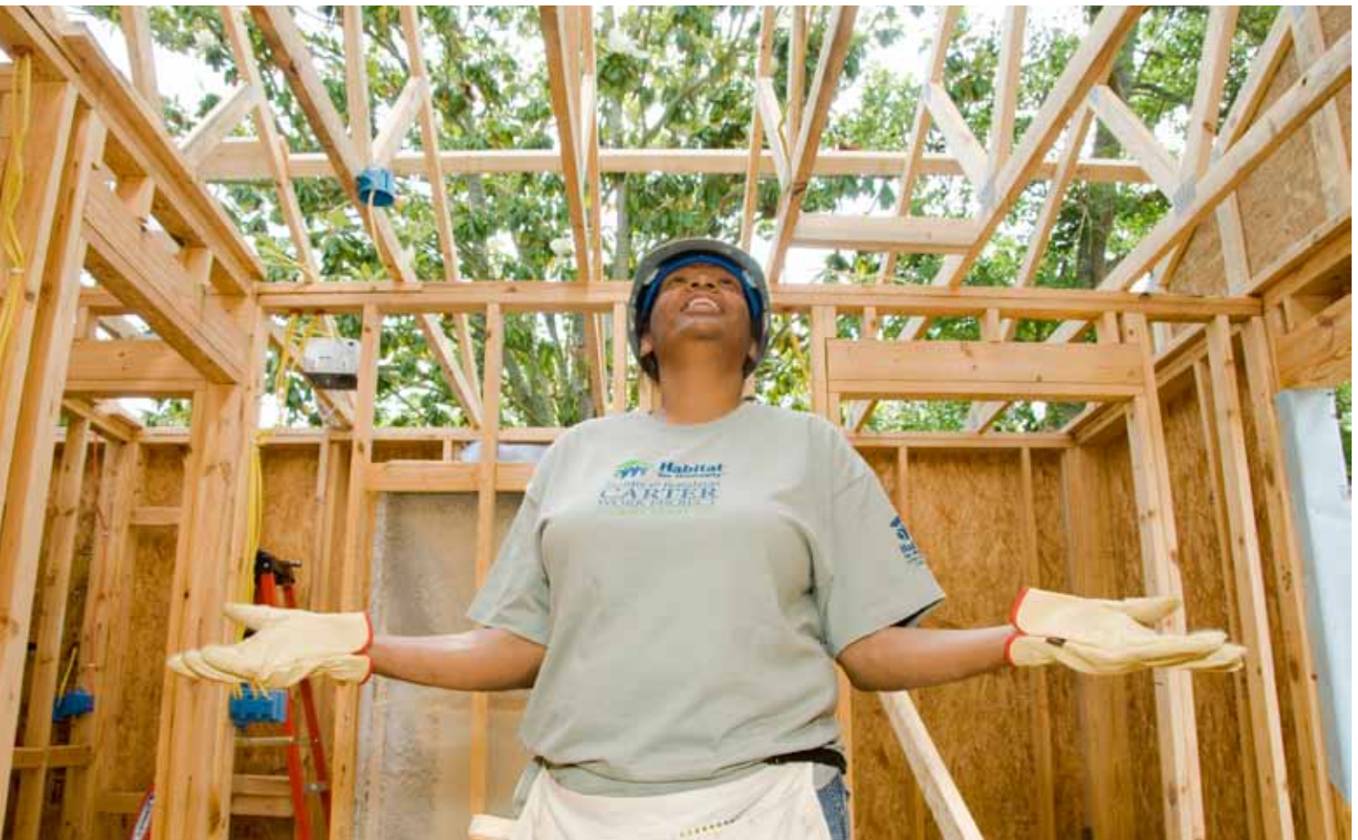
Christine Logan marvels at the progress on her future house in Pascagoula, Mississippi, during the 2008 Jimmy & Rosalynn Carter Work Project.
