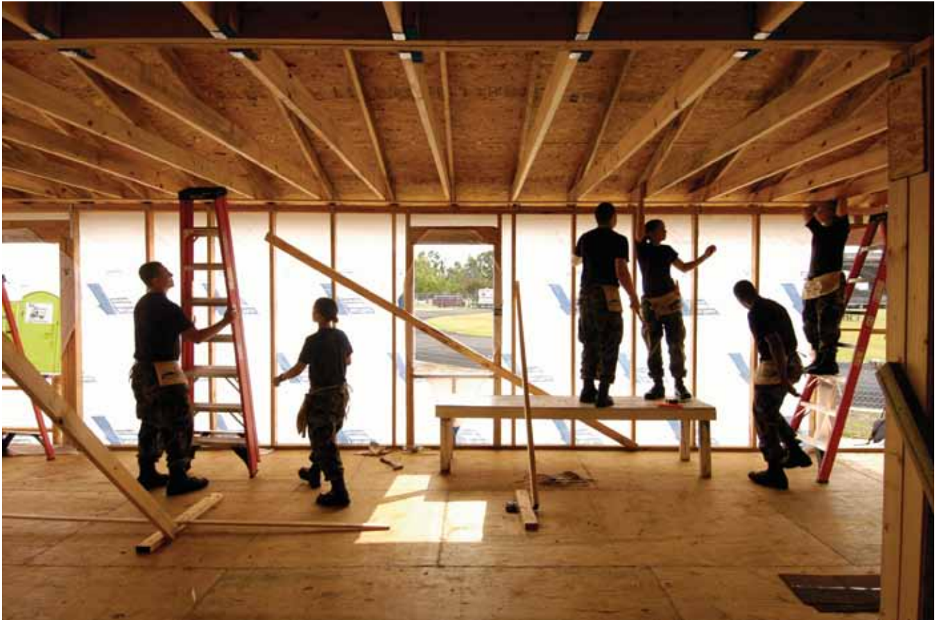
In 2006, U.S. Air Force personnel from Keesler field in Biloxi, Mississippi, help build temporary units in “Volunteer Village.”
