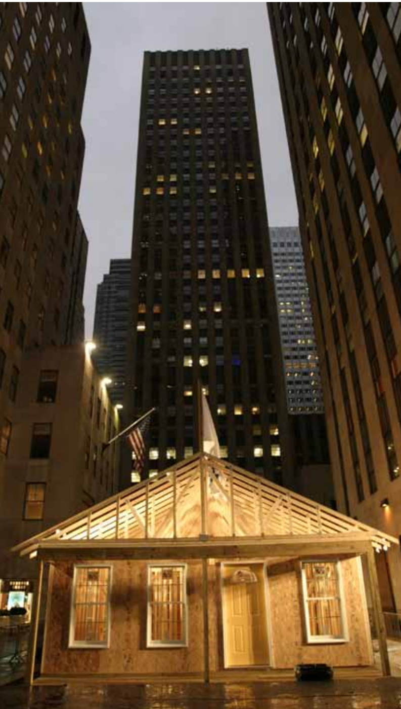
In late September 2005, Rockefeller Plaza in New York City becomes “Humanity Plaza,” as volunteers build houses for Habitat for Humanity’s Operation Home Delivery to help families displaced by Hurricane Katrina.
