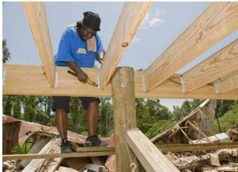
Homeowner Kiwana Thorton hammers on the foundation of a Habitat house in Slidell, Louisiana, as debris from a destroyed trailer still sits in the background.
