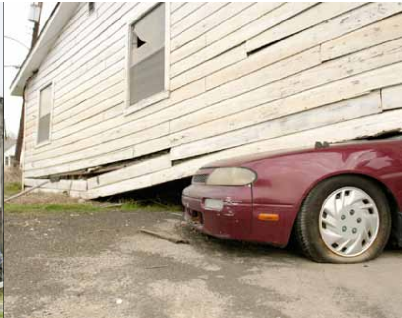
A car is crushed under a house after flooding in New Orleans' Lower 9th Ward.
