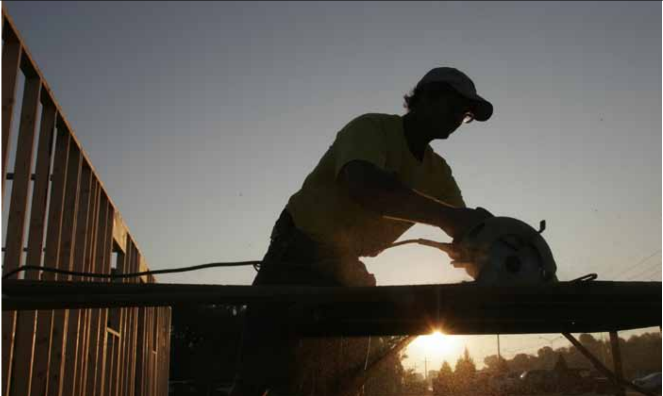
Mark Scott, then construction manager for Metro Jackson (Mississippi) Habitat for Humanity, cuts plywood as dawn breaks on Sept. 28, 2005. Among the earliest Habitat responders after Hurricane Katrina, Scott now works as construction director for the Bay-Waveland affiliate.
