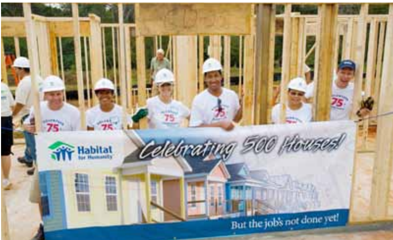
In November 2006—less than 15 months after Katrina and Rita—walls are raised on Habitat's 500th hurricane recovery home, in Mobile County, Alabama.
