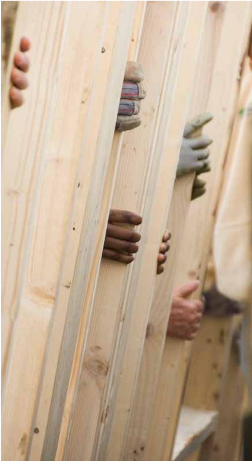
Volunteers raise the wall on a new home in New Orleans East. More than 2,500 people attending the 2008 NBA All-Star Game, along with NBA All-Stars, former NBA players and celebrities participated in projects throughout New Orleans for the "NBA Cares Day of Service."
